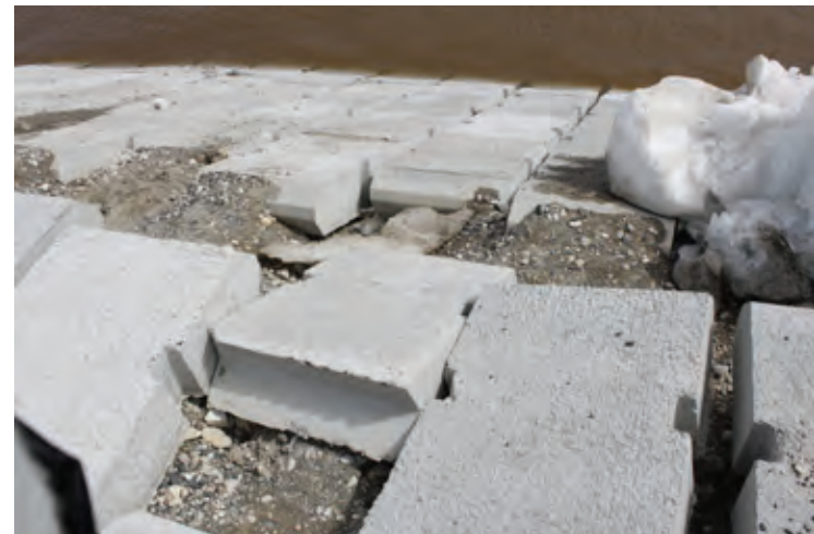
Fig. 29 - Many of the blocks along the lower edge have been dislodged by the massive ice chunks. None of the blocks are tied back to the dike, they just rest on the surface.
