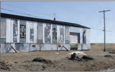
Fig. a2 - Abandoned old church
