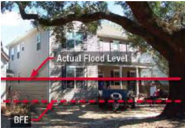
fig. 108: Flood Level Exceeded BFE
