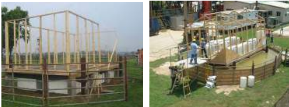
Figure 9: Full-scale testing of prototype buoyant foundation system. Construction of prototype; stability test showing floating platform tilted due to unevenly distributed sandbags representing imbalanced live load.
