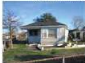
heavy structural damage
