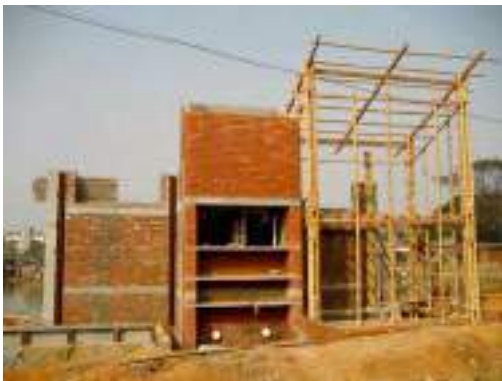
Day 46 – Brick work is finished and bamboo frame for one dwelling is started
