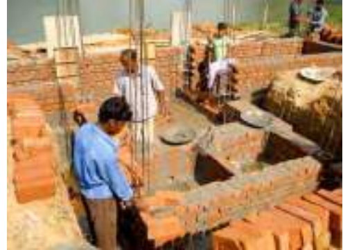
Day 10 – Brick foundation walls are started for water cisterns and composting latrine storage
