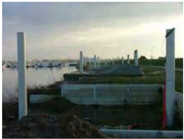
all components are ready to receive the first concrete box foundation for the amphibious house
