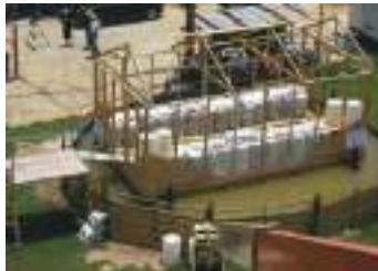
Students from Louisiana State University built a house frame with a buoyant foundation to test the floating house design. Photo courtesy of Elizabeth English
