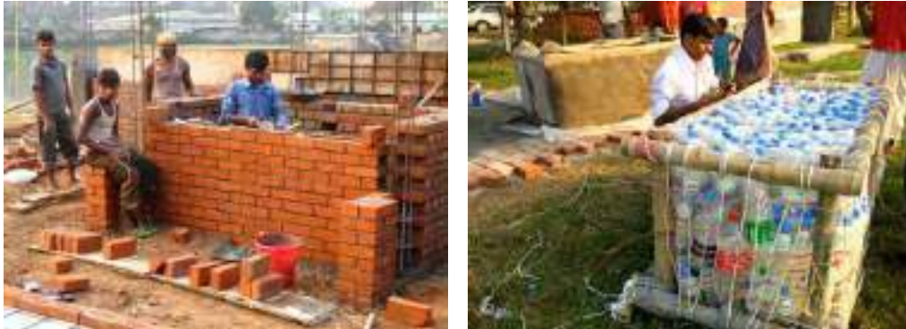
Figure 7: The LIFT House in Dhaka, Bangladesh. Concrete and brick base structure under construction; buoyancy block made of recapped, recycled plastic bottles.
