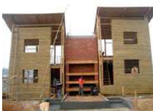
Day 66 – "You will notice in Photo25...the house on the right is higher than the left.. its floating!" (this has the recapped plastic bottle buoyancy blocks)
