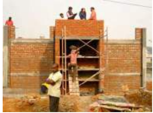
Day 32 – water cistern top slab and brick walls with concrete beams are finished
