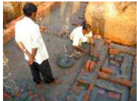
Starting the brick walls for the composting latrines and rainwater storage cisterns
