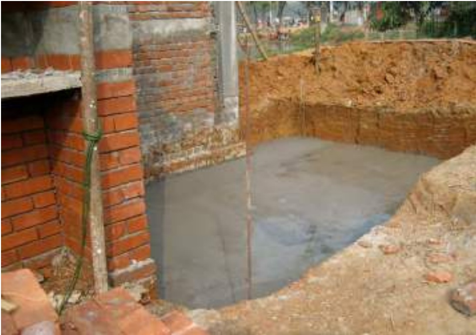
8.57. Layer of concrete on brick soiling on the bottom of the water bottle foundation dwelling holding tank
