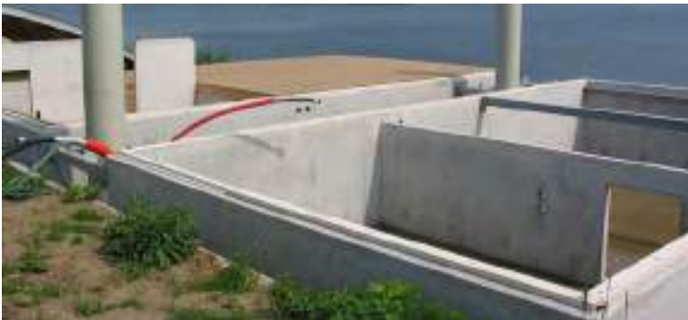
5.6. Concrete foundations, poles and flexible plumbing connections
