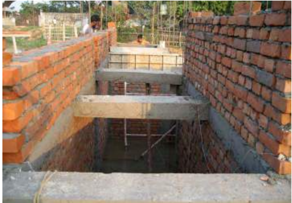
8.49. Lintels for lateral support inside the water cisterns in the service spine
