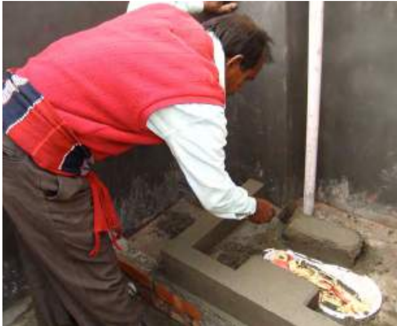
8.96. Custom latrine made to divert urine
