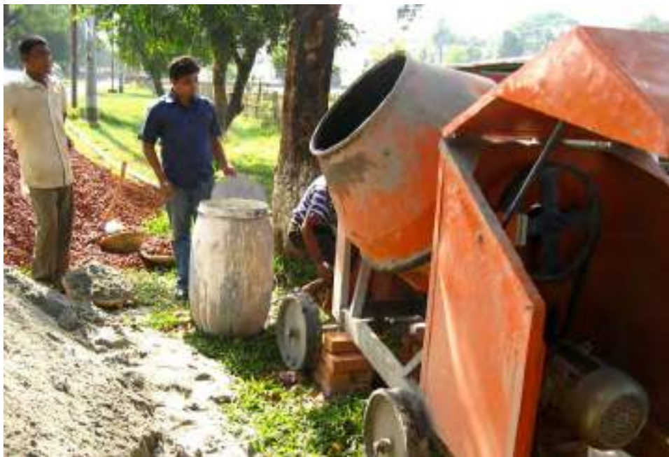
8.25. HBRI's concrete mixture used to pour floor slab of the service spine
