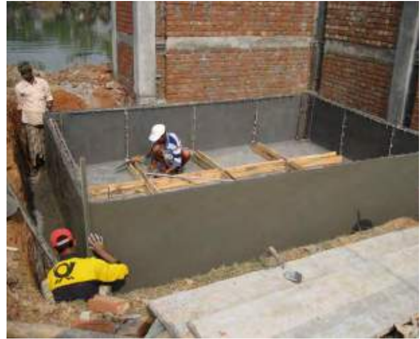
8.63. Cement mixture laid on both the outside and inside face of the foundation
