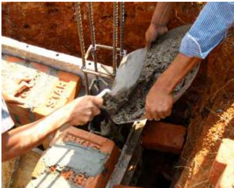
8.30. Concrete poured into gaps left for columns in the brick walls of the service spine
